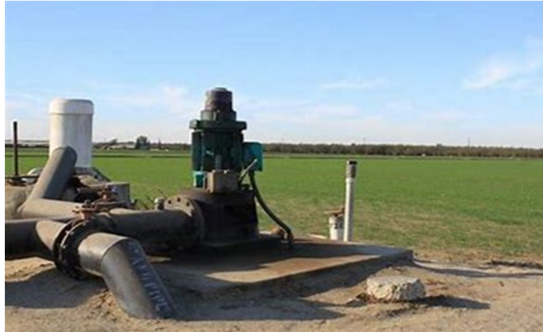
Groundwater Pumping Station
